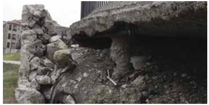
Water and its various forces are a common culprit leading to extensive deterioration and failure of retaining wall systems.
