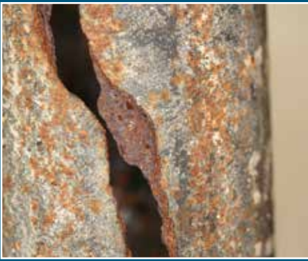
A. Cracked vent line
